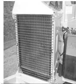
RADIATOR SCREEN - CLEAN FROM THIS SIDE
